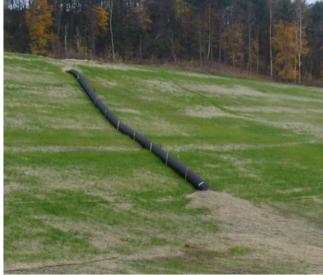
Figure 3.26 Temporary Slope Drain (Mass DEP 2019).
