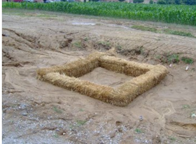
Figure 3.57 Straw Bale Inlet Protection (Indiana DEM 2007).
