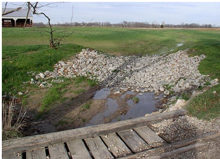
Figure 3.51 Grade Stabilization Structure (NRCS 2014).
