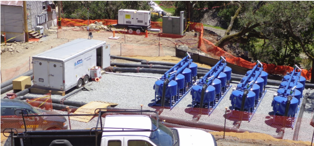
Figure 3.19 Active Treatment Systems Plant at a Construction Site (Active Treatment Systems 2019).
