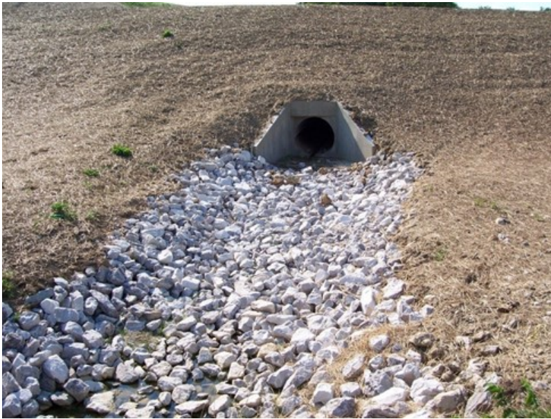
Figure 3.52 Riprap Outlet Protection (MN PCA 2016a).
